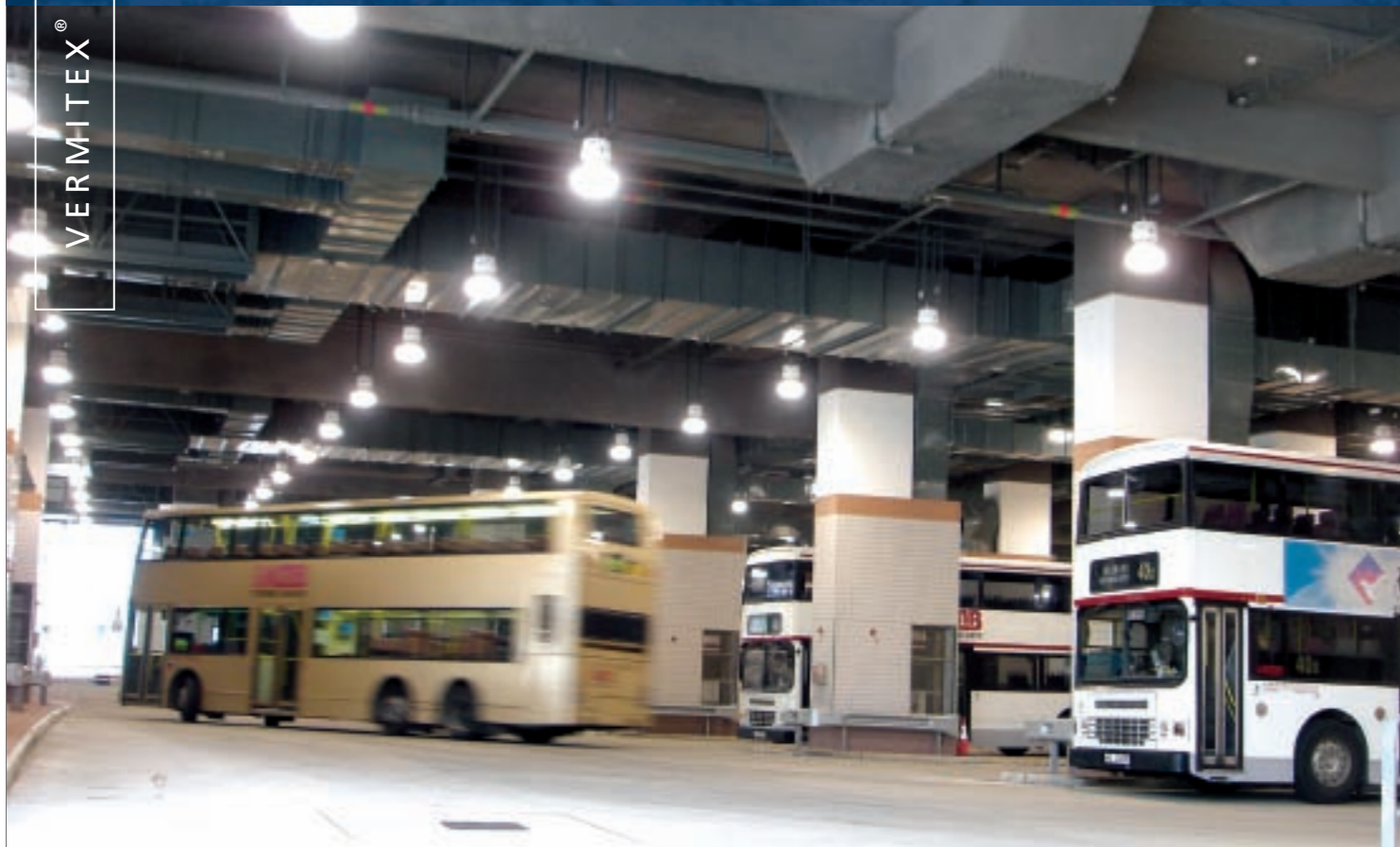
Vermitex® 'Acustico' in transport depot of the KCRC Wu Kai Sha Rail Station in Hong Kong.
